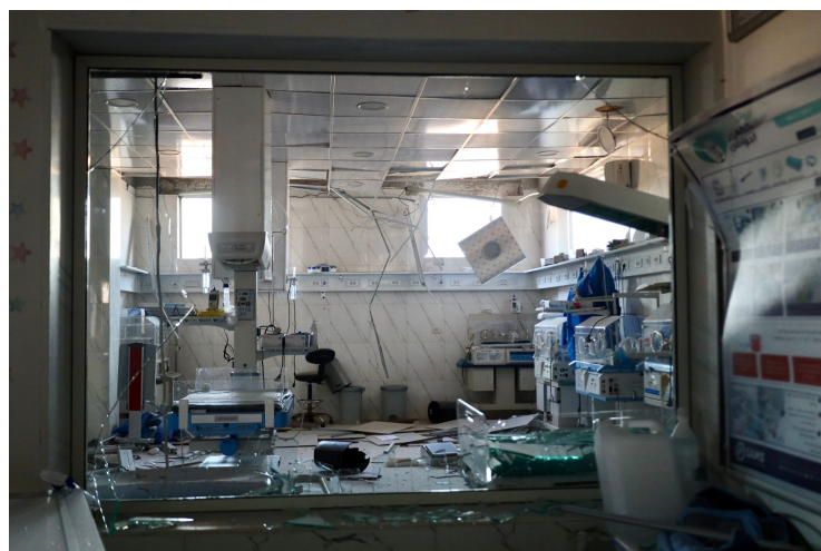
Damage to the Maternity Hospital in Idlib. © UNFPA/Syria
